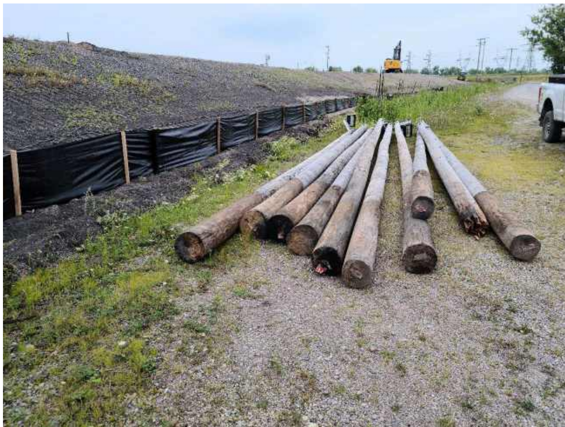
Photo 1: Power/Light poles Fisher removed from the south side of the Lined Impoundment.
