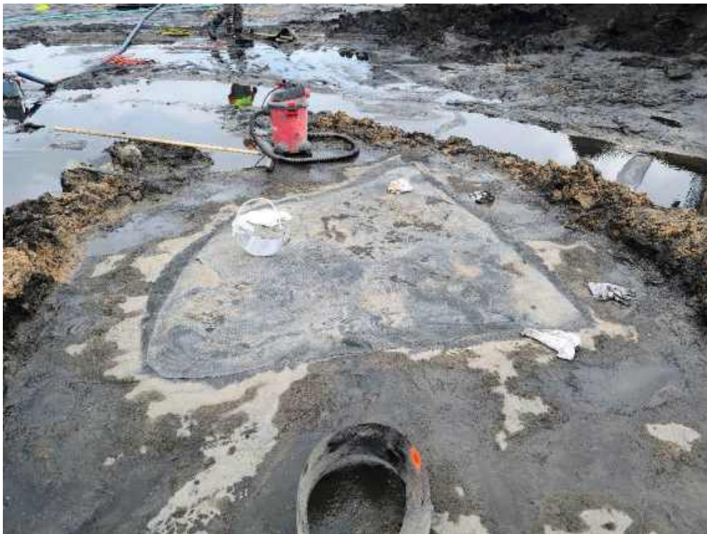
Photo 2: Fisher completes a repair to the primary geomembrane liner system in the Settling Basin.
