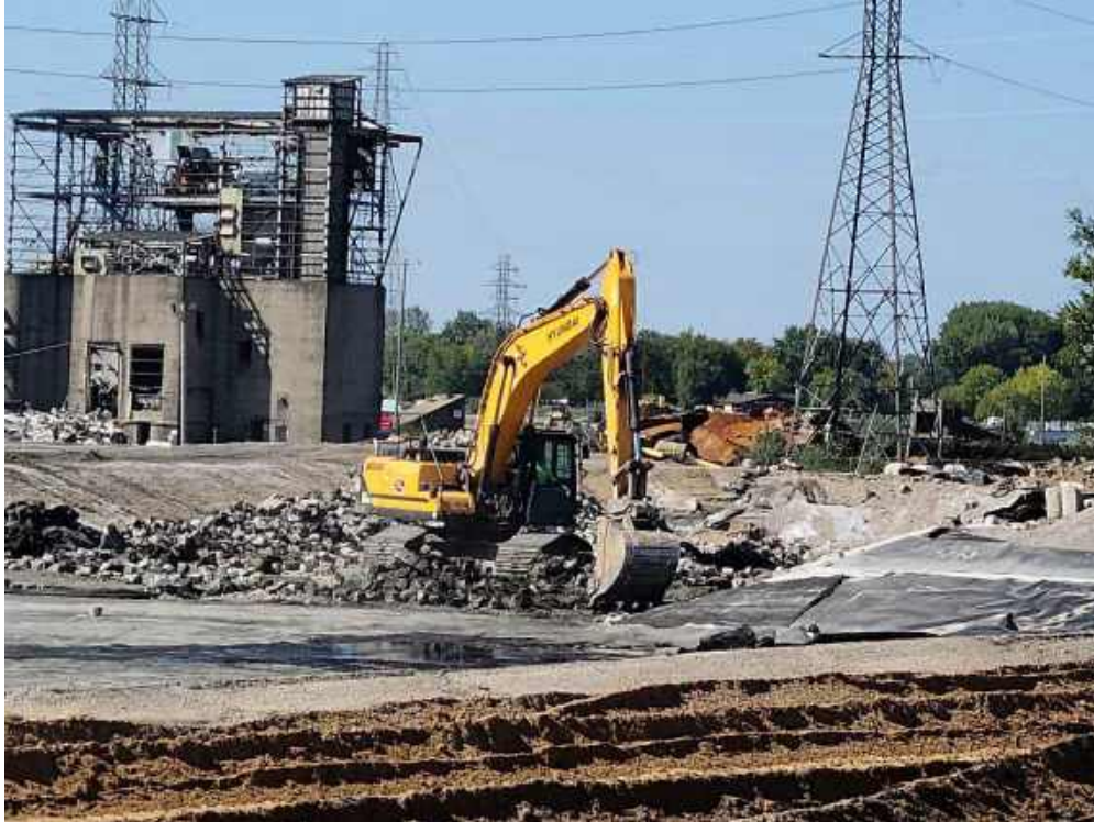
Photo 1: Fisher removing the concrete geoweb liner over the west end of the Settling Basin.
