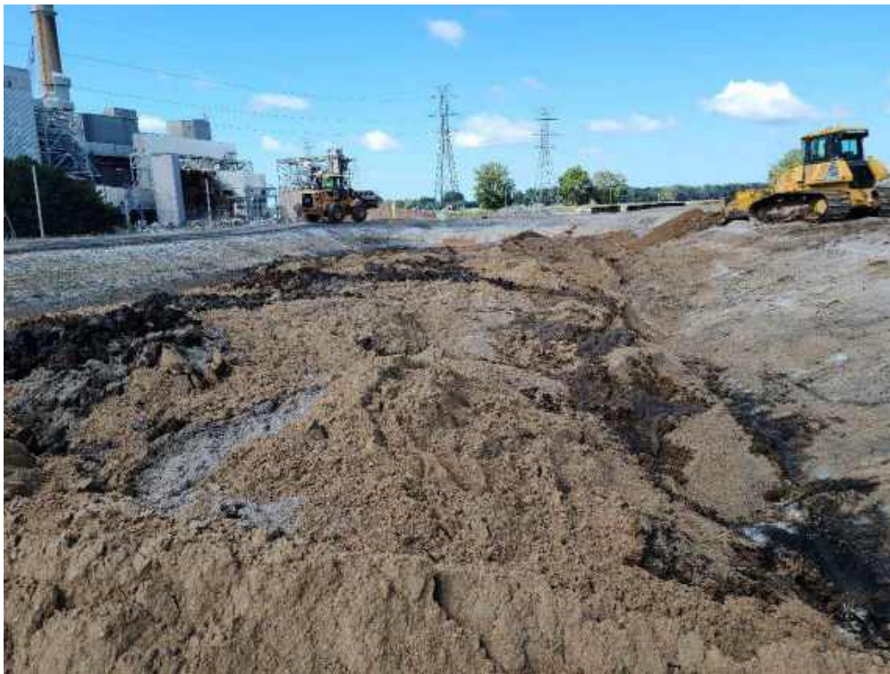
Photo 1: Fisher is mixing sand into the ash in the concrete-lined portion of the Settling Basin.
