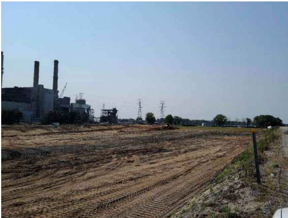
Photo 2: Fisher grading the Settling Basin after the liner systems have been removed.
