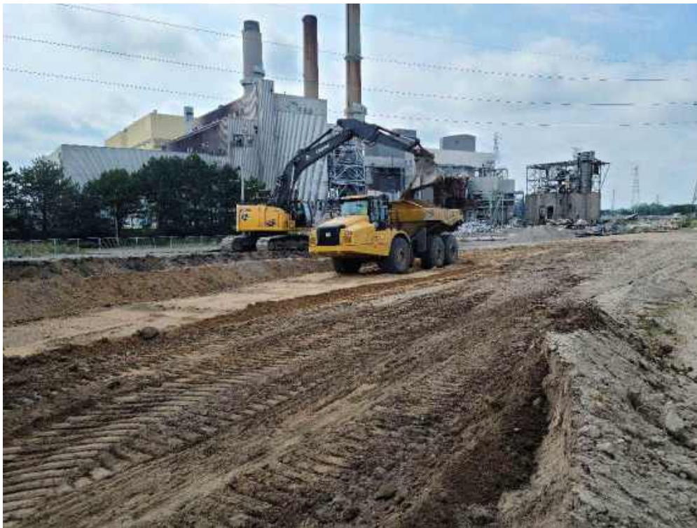
Photo 1: Fisher excavating excess berm material from the west end of the Lined Impoundment.
