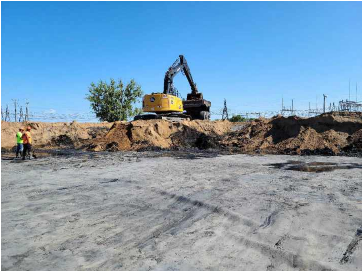
Photo 2: Fisher loading out ash/sand mix above the primary liner of the Settling Basin.
