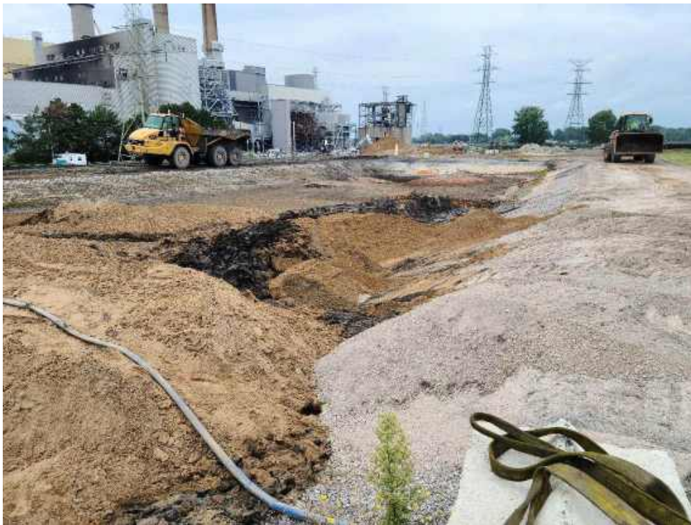
Photo 1: Fisher starts mixing sand in with the ash in the concrete-lined portion of the Settling Basin.
