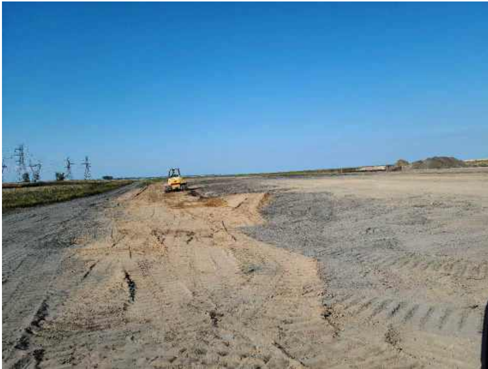
Photo 2: Fisher covering the placed ash located adjacent to the north/south road in the Weadock Landfill.
