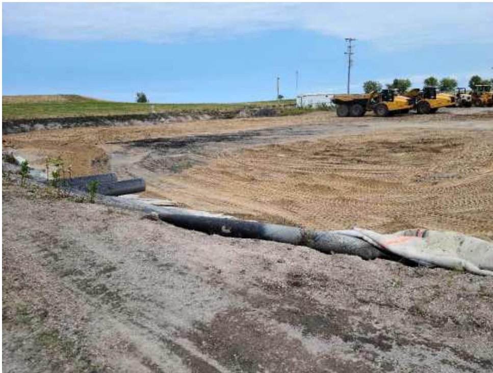
Photo 2: The Polishing Basin with most of the geomembrane liner and GCL removed.
