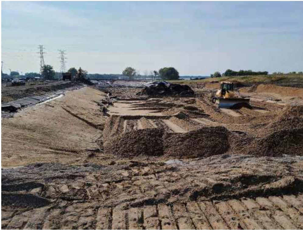
Photo 1: The removal of the primary and secondary liner systems from the Settling Basin.
