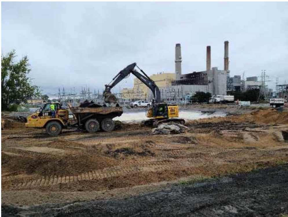
Photo 2: Fisher loading geomembrane liner and GCL for disposal in the JCW Landfill.
