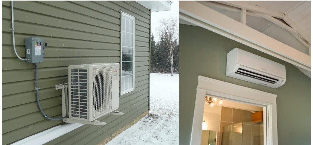
Figure 23: An example of a ductless mini-split heat pump outdoor compressor mounted to stay above the snow and a wall-mounted indoor fan coil. 35
