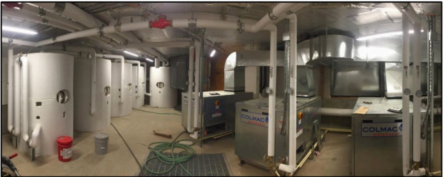
Figure 19: Ecotope Case Study "RCC" system for 194-unit Multifamily building, using best practices in central heat pumps for domestic hot water, from ACEEE presentation by Shawn Oram. 30
