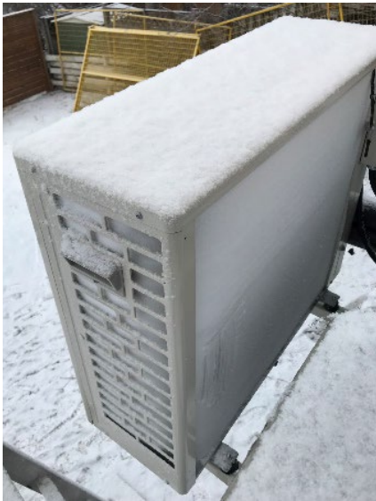
Figure 21: The Eco2 heat pump water heater compressor working outside in 5°F (-15°C) weather. 33
